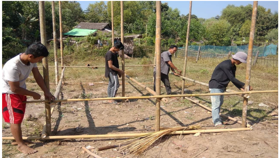
Building temporary houses in the forest for the internally displaced people of Myanmar
